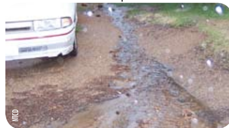
Runoff cuts side yard channel
